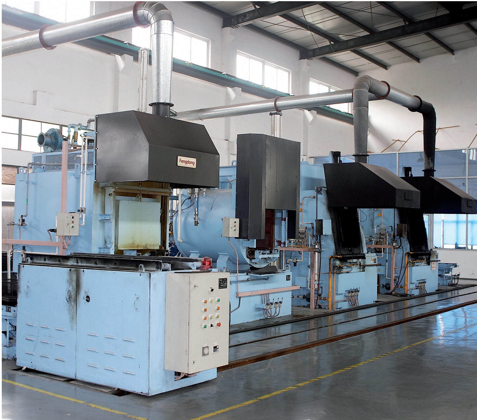
Vacuum Cleaning/Carburizing Quenching Furnace
